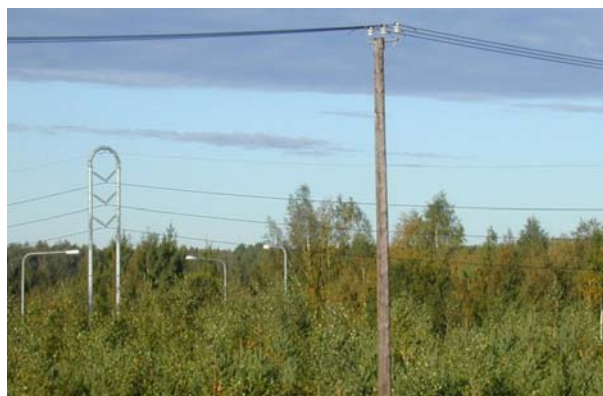
Figure 1. MV and HV covered conductor lines in Tuusula, Finland.
