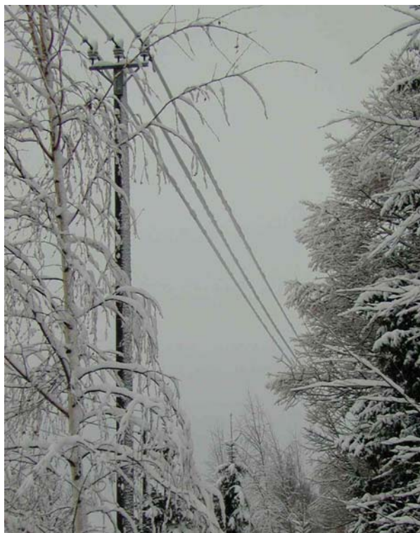
Figure 2. Typical condition faced by MV lines in Finland during wintertime.
