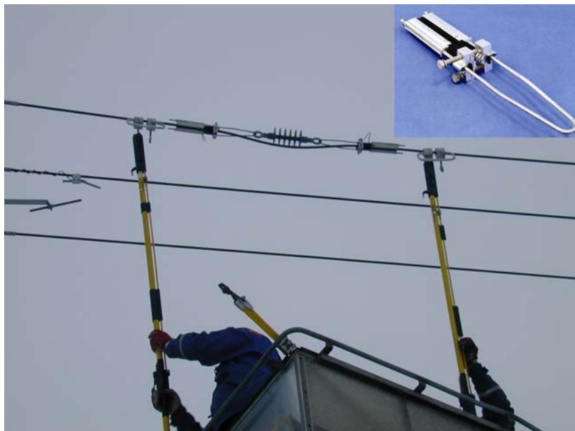
Figure 5. Live line disconnection point is made to MV CC line.
